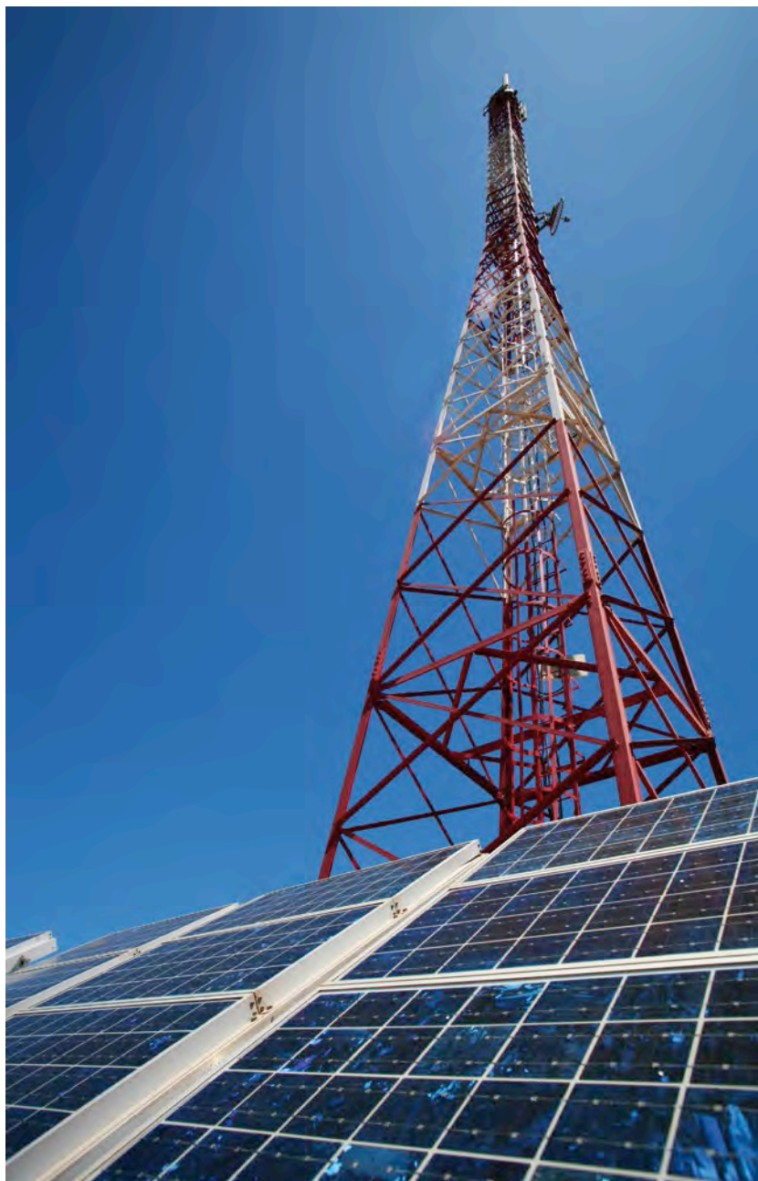
A tower company in Africa has to take over all the running of the passive infrastructure: the generators, the batteries and the air-conditioning. Picture: Ericsson
